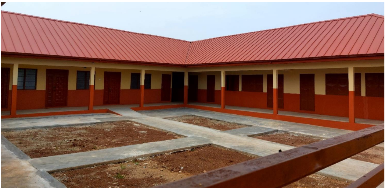
Photo 17: Construction and furnishing of 1No. 6-Unit JHS Girls Model with Ancillary Facilities at Nanton
